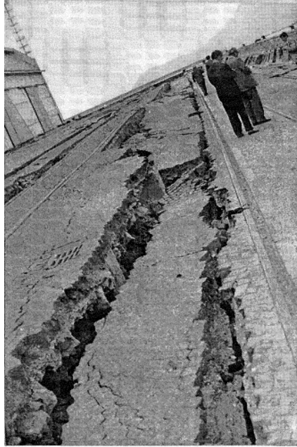
FIG.I.22 - Phenomena of horizontal displacement in Tivari port (Montenegro).
