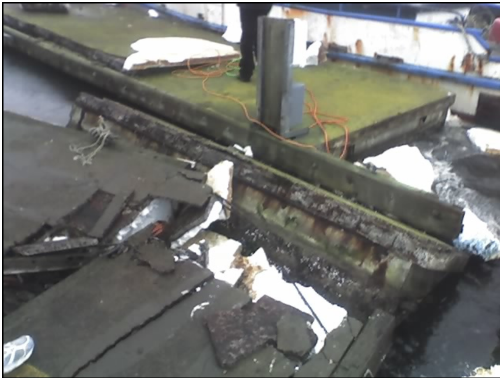
Photos of Damage to Crescent City Harbor.
